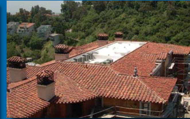
The Bel Air Project • TPO, Clay Tile & Copper Gutter System • Bel Air CA
