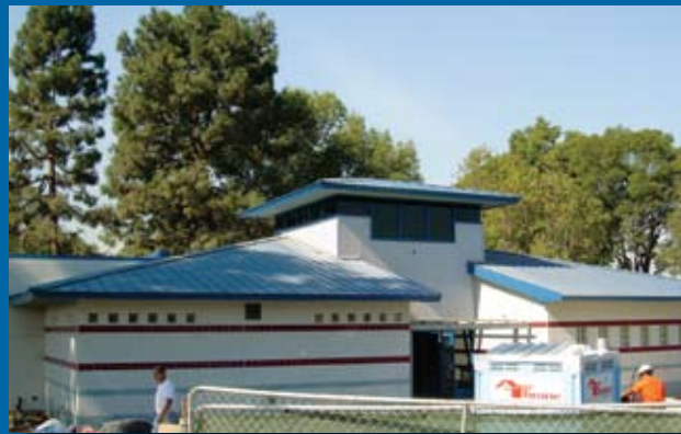
Admiral Kidd Community Center • Metal Siding, Roof & BUR • Long Beach, CA
